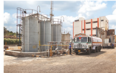
Tank Farm for Raw Materials.
